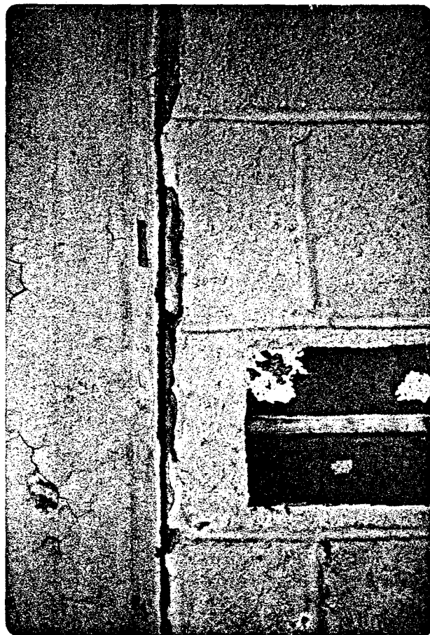
Fig. 65 Column Movement, EW Stairway Wall, during E.W. Shaking
