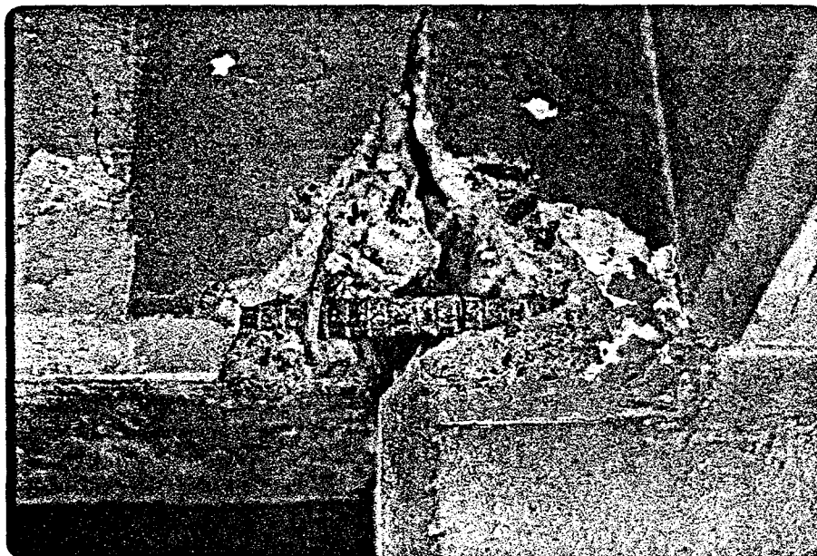
Fig. 72 East End of Beam B-4 Level 2, After E.W. Shaking
